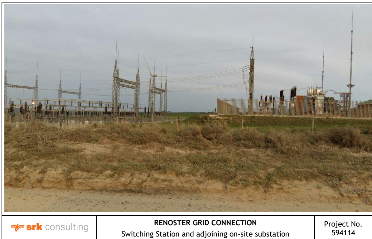
Figure 2-11: Example of a switching station (left) and adjoining wind farm substation (right) on the Kouga Wind Farm
