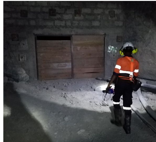
Closed regulators requiring sealing
