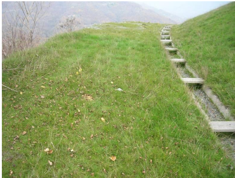
Fig. 6: Runoff collection channel on a top berm. Grass has already covered the remodeled sterile fills.
