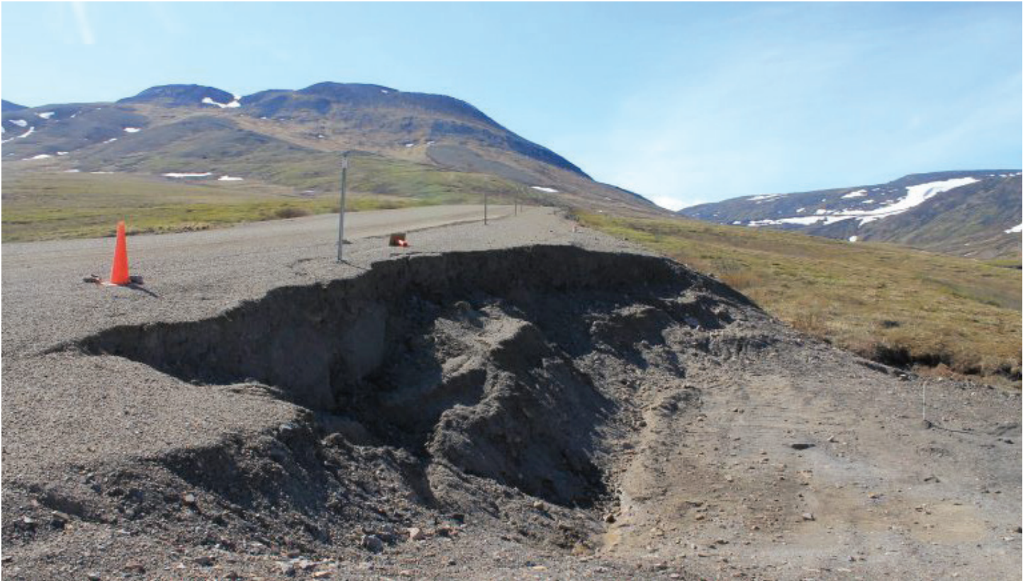
Highway embankment impacted by perpetual thaw of permafrost in the Northwest Territories. CREDIT: KISA ELMER, SRK CONSULTING (CANADA), INC.
