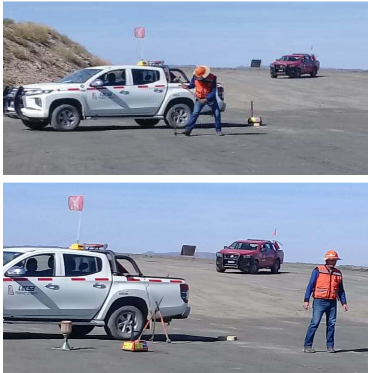
Figure 13 Quality control of the pilot stack including sand cone and a nuclear gauge
