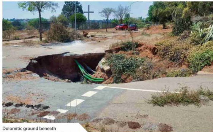
Dolomitic ground beneath infrastructure developments increases the risk of subsidence and sinkholes
