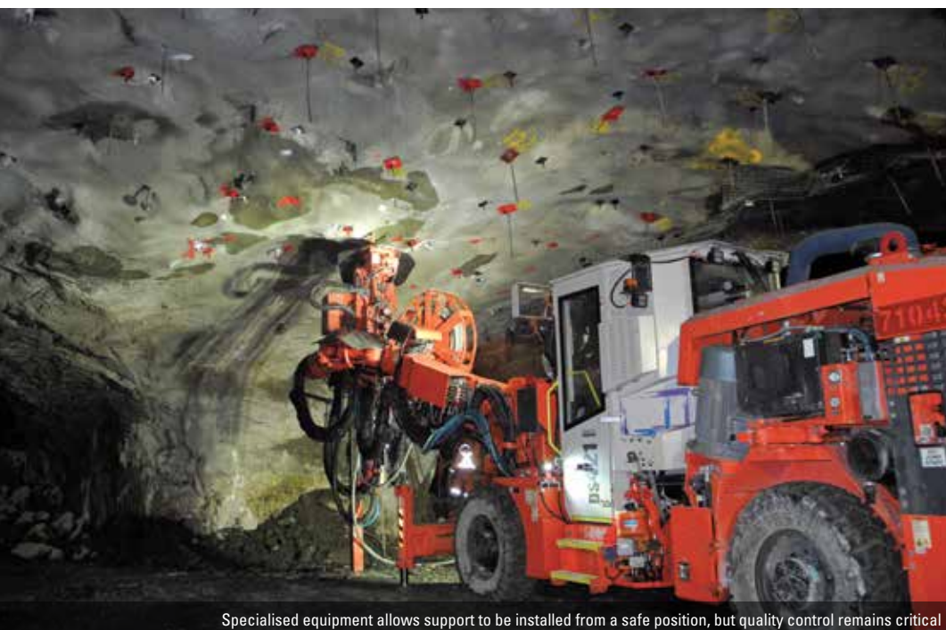
Specialised equipment allows support to be installed from a safe position, but quality control remains critical
