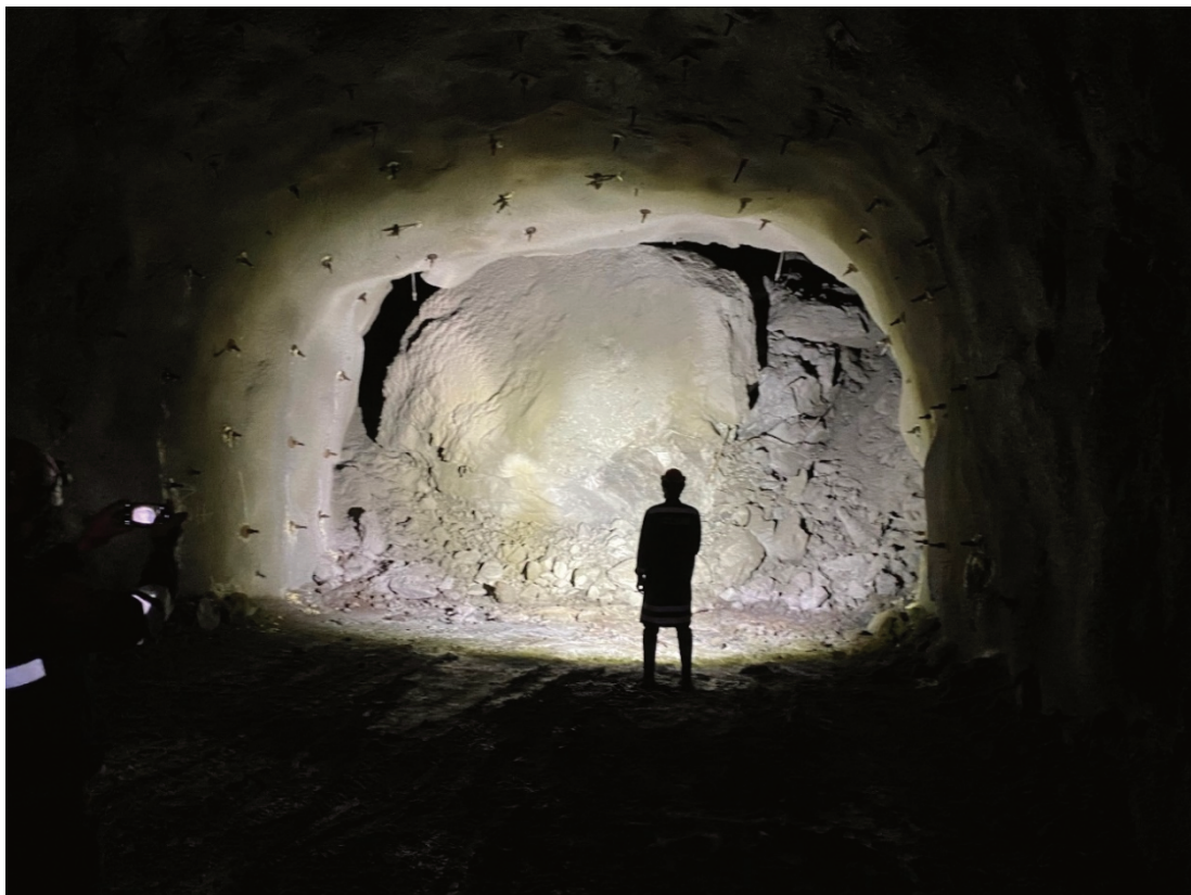
Figure 3 Level 1079, Y202 crosscut looking west, fragmentation and oversized boulder
