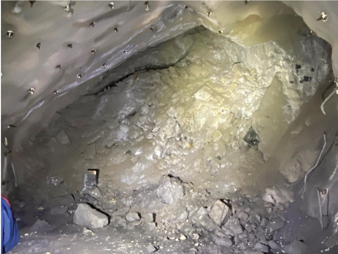
Figure 4 Level 1079 crosscut Y204 looking west, complete sealing of development
